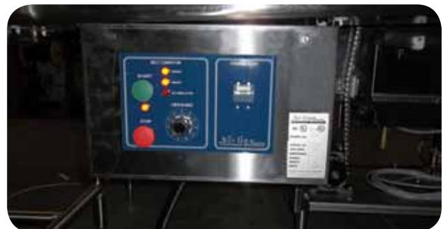
Control panel with variable speed control
