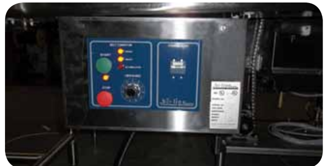
Control panel with variable speed control
